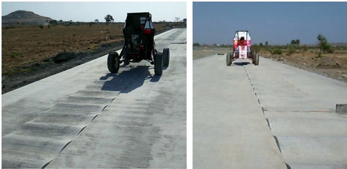
Figure 4.46: Low (left) and high severity (right) one-sided washboard tracks.
