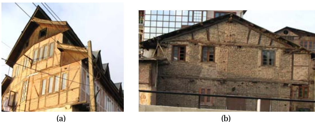
Figure 1 Traditional masonry for proven earthquake resistance: (a) Dhajji-dewari system of timber laced masonry for confining masonry in small panels and (b) Taq system of embedding timber thick walls
