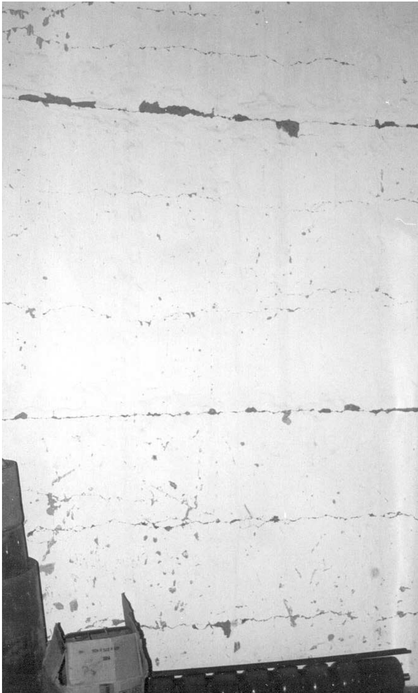
Figure 2. Cracks are 'through' the shell thickness as seen from inside the shaft of 1000 kL Anjar Nagar Palika Tank.
