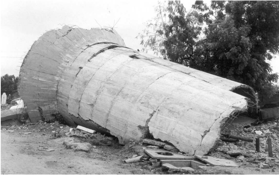
Figure 4. Collapsed 265 kL water tank in Chobari village about 20 km from the epicenter. The tank was approximately half full during the earthquake.
