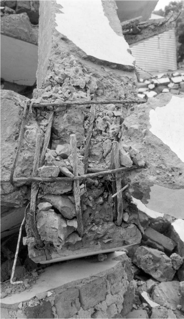
Figure 6. Poor detailing of column-brace joints for Manfera tank.
