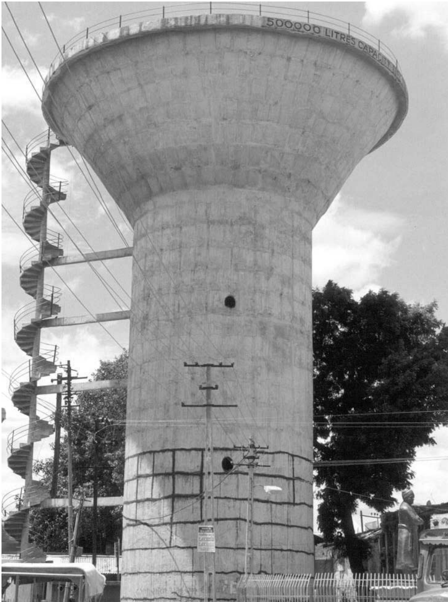
Figure 3. Flexural cracks in staging of 500 kL tank being repaired by injecting epoxy. This tank in Morbi, 80 km away from the epicenter, was empty at the time of the earthquake.
