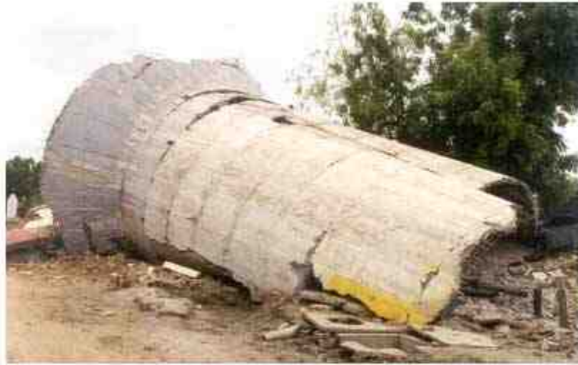
Figure 1: Collapsed 265 kL water tank in Chobari village about 20 km from the epicenter. The tank was approximately half full during the earthquake.
