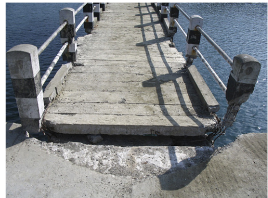
Fig. 5. Pounding damage to jetties in Middle Andaman, at the construction joint of approach jetty and berthing jetty at Sagar Dweep.
