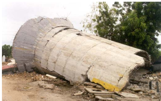
Figure 2. Collapsed 265 kL water tank in Chobari village about 20 km from the epicenter. The tank was approx. half full during the earthquake.
