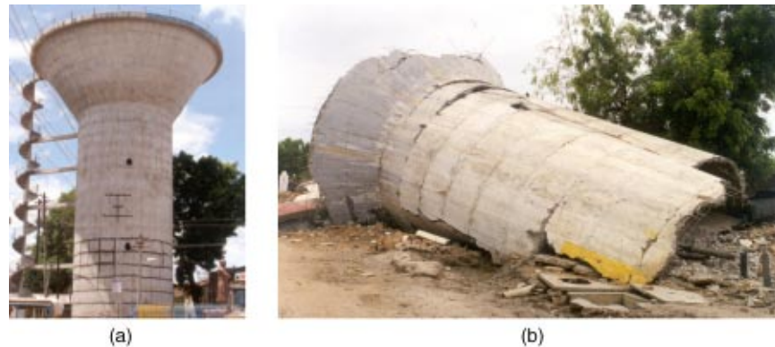
Figure 1. (a) Flexural-tension cracks in support shaft of 500 m 3 tank being repaired by injecting epoxy in Morbi, 80 km away from epicenter of the Bhuj earthquake; and (b) collapsed 265 m 3 water tank in Chobari village, about 20 km from the epicenter.
