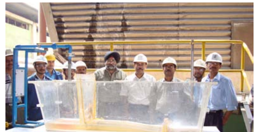
Prof. Mazumdar with JSPL engineers celebrating installation of slab caster water model tundish in SMS of JSPL . Raigarh works:
