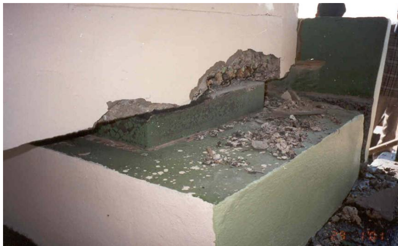
Fig. 4 Girder shifted in the longitudinal direction with loss of seating during shaking
