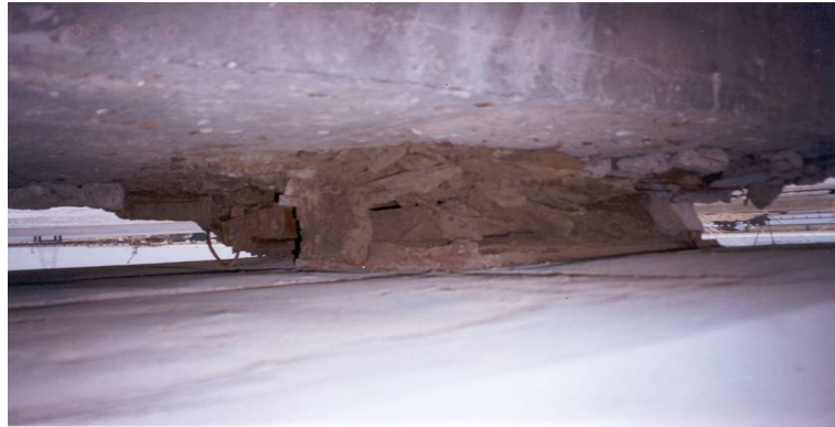
Fig. 3 Surajbari Old Bridge: Metallic bearings destroyed during earthquake
