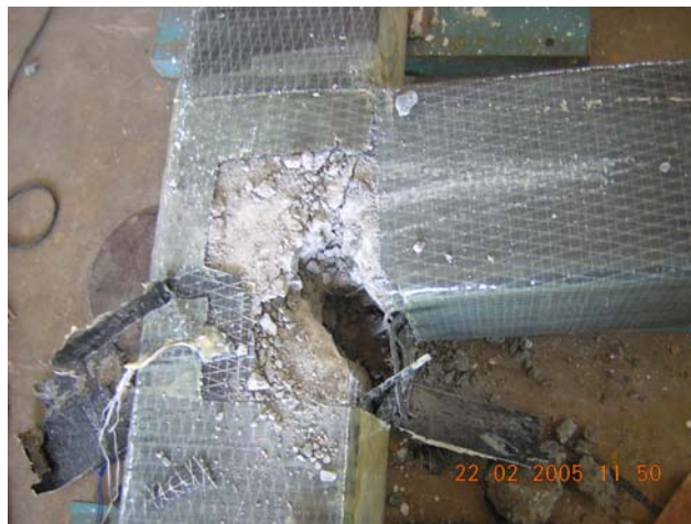
Fig. 13 Typical failure of beam-column joint with CFRP
