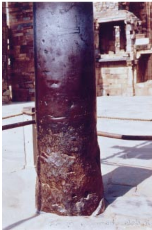
Figure 4. Hammer marks clearly visible where the rough region changes to a smooth region. This rough region was buried underground when the pillar was located originally in a Hindu temple.
