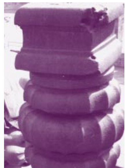
Figure 13. A fractured section of the top pedestal, indicating that it is a single piece of wrought iron.
