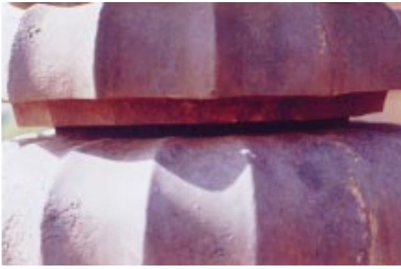
Figure 10. A close-up view of the joint between the 20 sided circular disc and the one above it.
