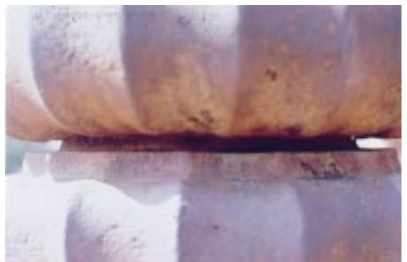
Figure 9. A close-up view of the joint between the 16 sided circular disc and the one above it.
