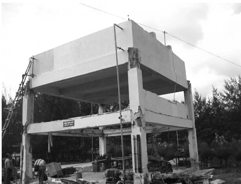
Figure 14. Out-of-plane failure of an infill wall and formation of a plastic hinge at the beam-column joint of a freshwater tank (50 kL capacity) at Suryachakra powerhouse in the Bamboo Flat area in South Andaman Island (photo: D. Rai).
