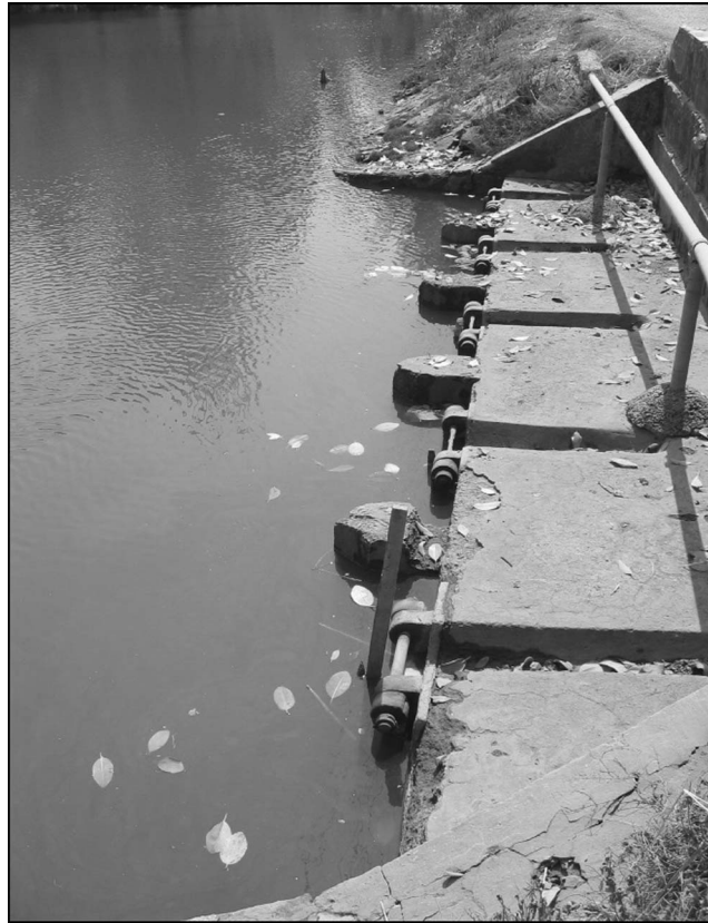
Figure 9. Damaged sluice gates under the South Andaman Island Trunk Road (photo: M. Yashinsky).
