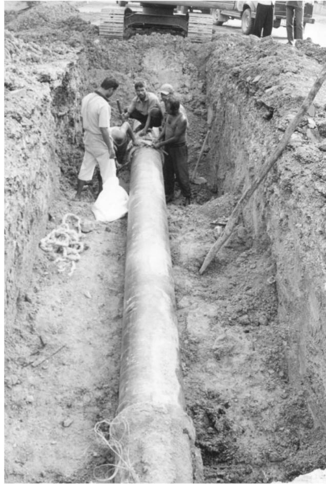
Figure 6. Damaged pipeline being attended to near the water treatment plant in Port Blair (photo: S. Dash).
