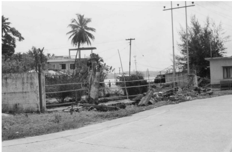
Figure 3. Collapse of the Suryachakra Power Plant masonry boundary walls at Bamboo Flat in South Andaman Island (photo: G. Mondal).
