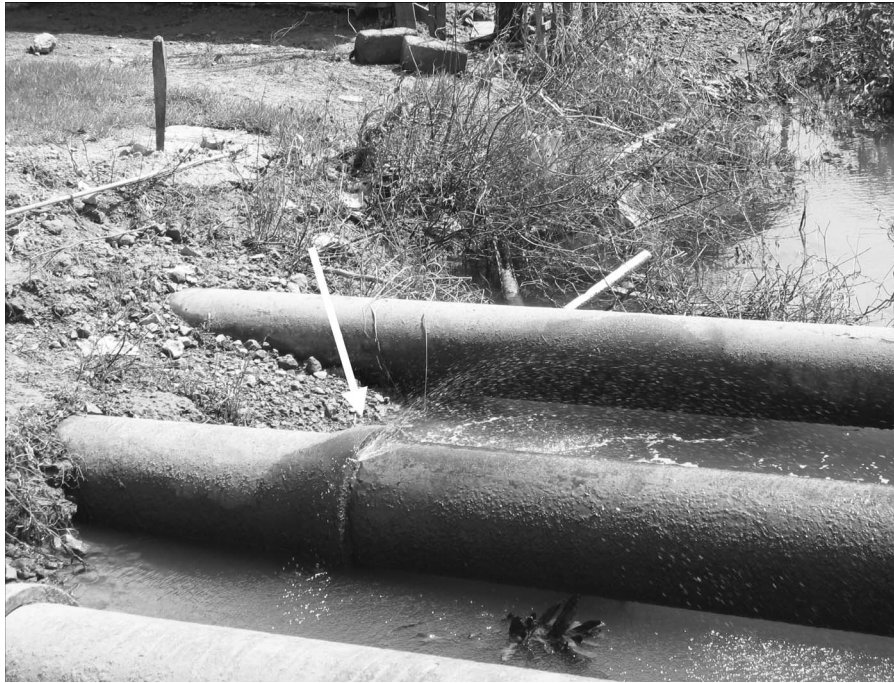
Figure 8. Water main leaking along the South Andaman Island Trunk Road (photo: M. Yashinsky).
