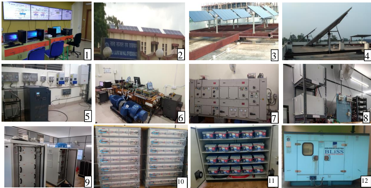
Fig.2: Photo of 1)Control Center, 2)100kW PV plant, 3)ThinFilm PV array with Single axis tracker, 4) Crystalline PV array with Dual axis tracker, 5) Hybrid and Grid-tied PV inverters, 6) Wind turbine-emulator & generator system, 7) HMG Interface panel, 8) Converters for Battery, SC and FC, 9)FC system with Electrolyser and H2 tank, 10)Battery Bank, 11) SC bank, 12) Diesel generator
